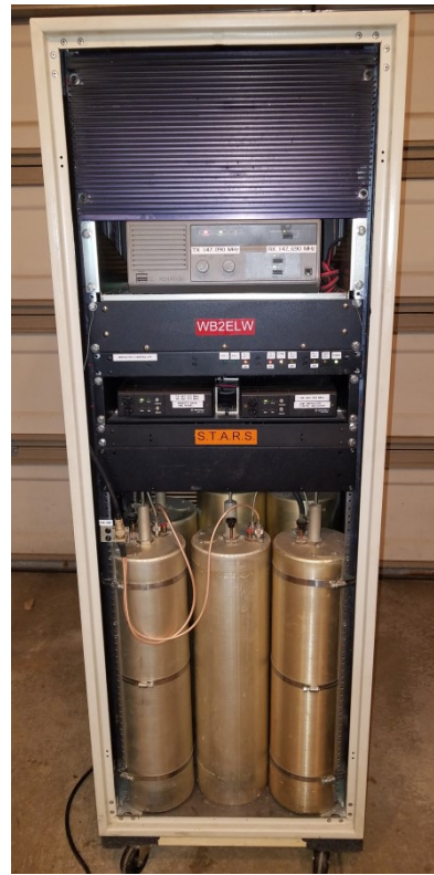
Figure 3: New Colden Repeater
