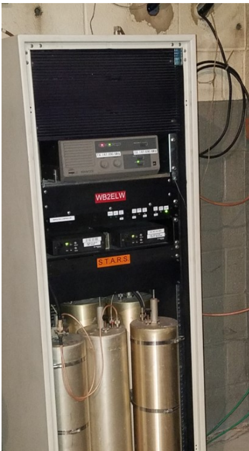
The New Colden Repeater
