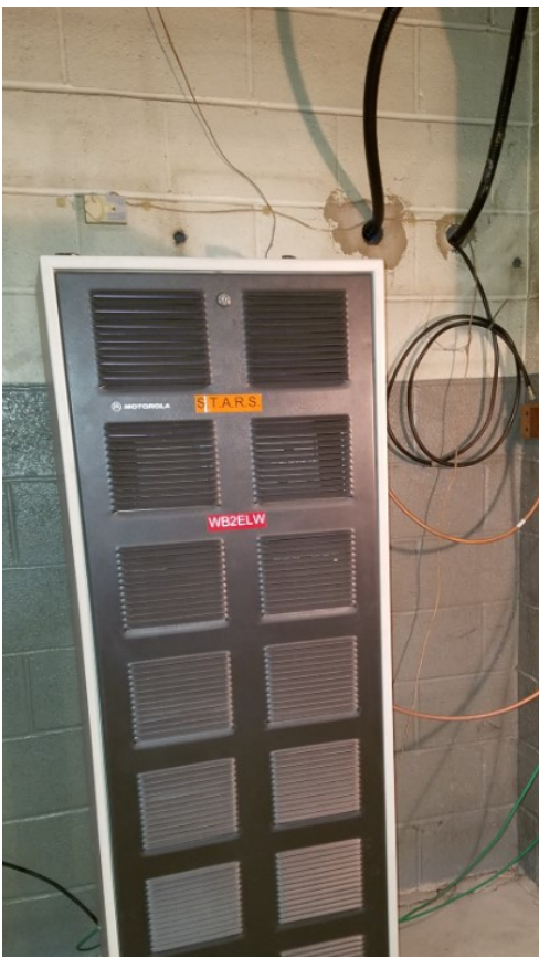
The New Colden Repeater
